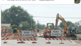
REPAIRS TO WEST 15TH STREET UNDER WAY Construction workers are working on repairs to West 15th Street. The project is expected to be completed by the end of the year.
